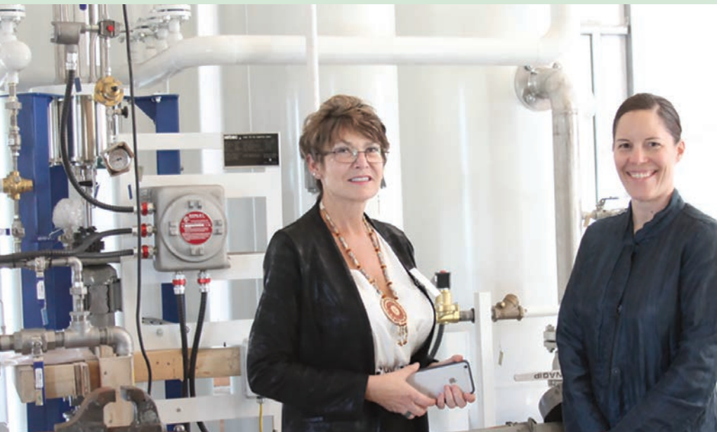
Blue Lake Rancheria Vice Chairperson Arla Ramsey and Energy Director Jana Ganion survey the progress of the Tribe's biomass-to-fuel cell power plant, scheduled to go online this spring. Photo from Jana Ganion, Blue Lake Rancheria, NREL 32766
